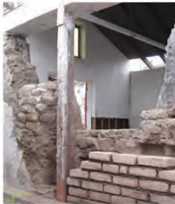
The barn was extensively remodeled in the 1970s, including CMU / concrete infills in damaged adobe walls, and installation of a concrete bond beam that changed roof lines and exposed adobe walls to additional damage.
