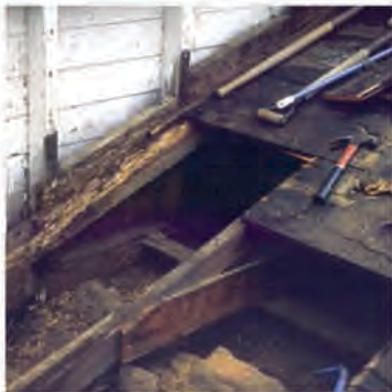
Failure of the roof covering in several places exposed roof framing and adobe walls to water damage.
