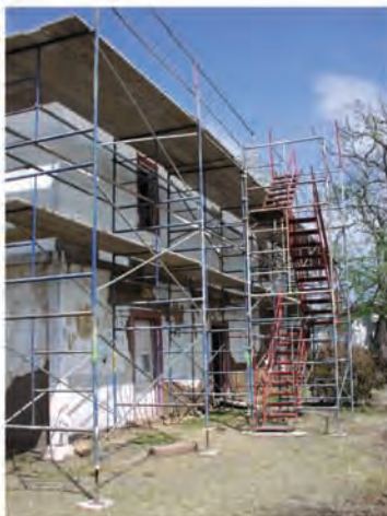
Scaffolding was set for the installation of seismic retrofit elements prior to reconstruction of the porches.
