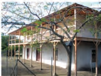
The porches were reconstructed of old-growth Douglas fir to match the original construction. Above are the reconstructed porches just prior to the installation of handrails.
