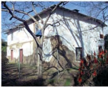
The loss of the porches exposed the adobe walls to weather damage, particularly at their bases, and eliminated the lateral support needed for seismic stability.
