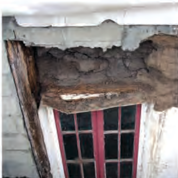
Failure of roof flashings and the exterior stucco resulted in partial wall collapses and the decay of wood lintels over windows and doors.
